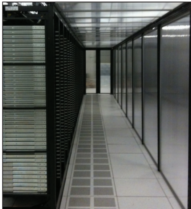
With cold-aisle containment, the cold row is capped at the tops of the cabinets and across the aisle, and doors are installed at the ends of the row to contain the cold air.
